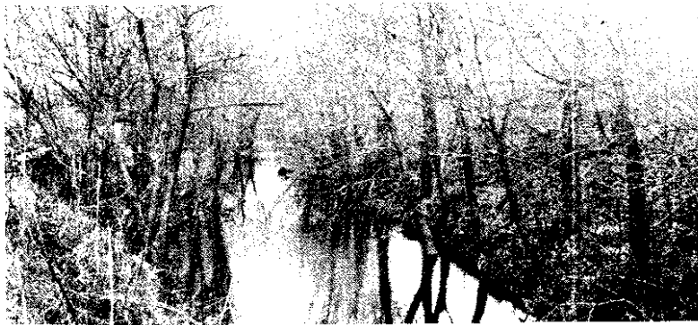
Kaskaskia Mutual Dredged Channel near Bondville, Illinois. Approximate bottom width 10 feet. Picture taken April 1925.
